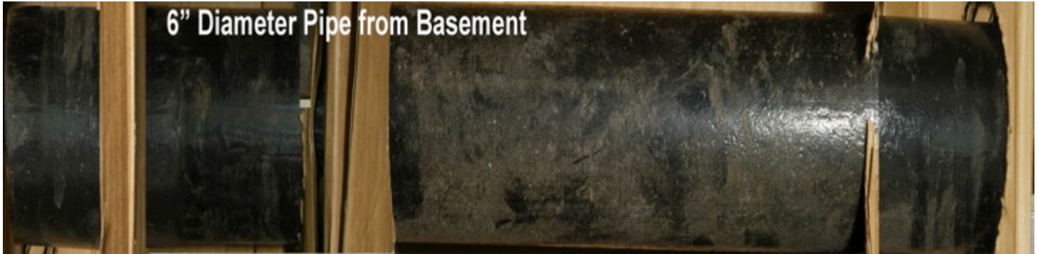
Photo 2-1 One section of black pipe
